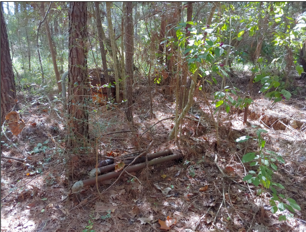
18. Piping associated with abandoned natural gas well.
