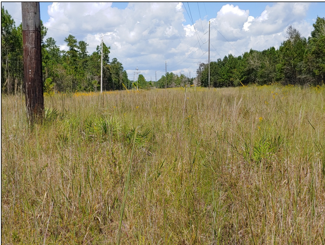
10. Electric transmission line on southern portion of Seven States property.
