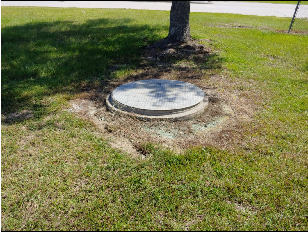
13. Likely sewerage lift station on southern boundary of Thian property.
