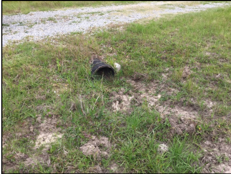
Photograph of stormwater drainage from railroad adjacent to the east of the property
