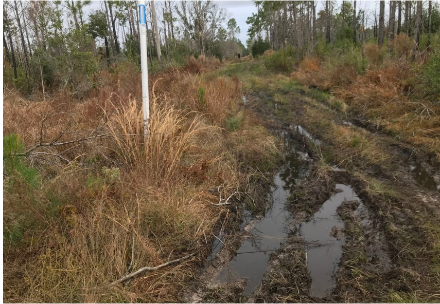
Photograph 2 – Standing Water at Gas Pipeline Easement Near Boring S-4
